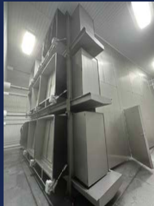
Three individual evaporators allow sequential defrost
