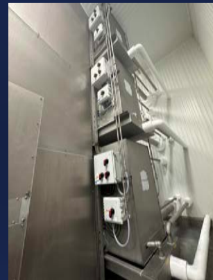
Factory wired UL listed panel, motors wired to individual disconnect.
