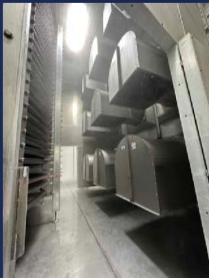
Fan tubes are tilted at a slight angle to increase air intake
